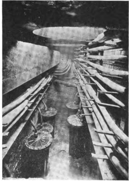
Loading manhole, showing loading coil cases, racking of cables, and at far end, cables entering ducts
