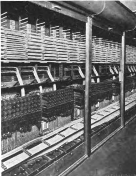
Rear view of toll switchboard
