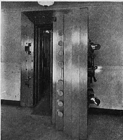
The fifteen-inch rectangular entrance to the security and safe deposit vault of the Title Guarantee and Trust Company, 7 Maiden Lane, New York. This vault has an eighteen-inch wall, reinforced with the well known type of rivet grip reinforcing—two and a half inches of which is composed of torch-resisting metal. This vault was recently installed by the York Safe and Lock Company of York, Pa.
