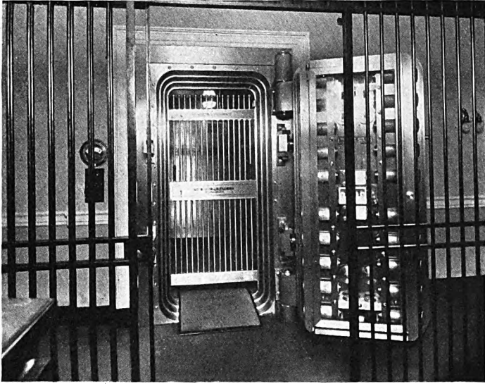
The vault work for the Union Trust Company of East Greenwich, R. I., furnished by the Mosler Safe Company, New York, consists of a 12 inch vault door, heavy steel lining, deposit boxes, etc. The vault is a two-story affair with deposit boxes on the street floor and the storage vault in the basement. Stairs on the inside of the vault connect the first and the basement story
