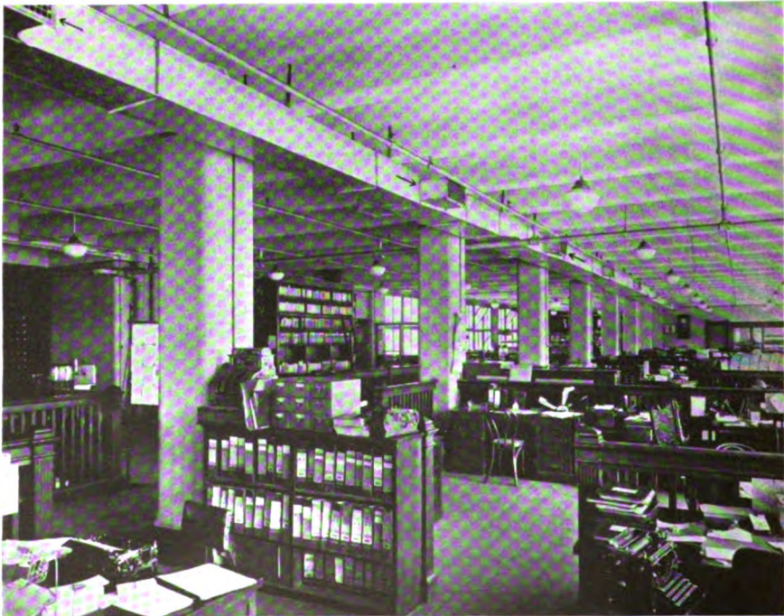
Showing arrangement of duct work in office, arrows indicating the registers through which fresh air is distributed. This system is especially applicable in old buildings where there is no central ventilating system
