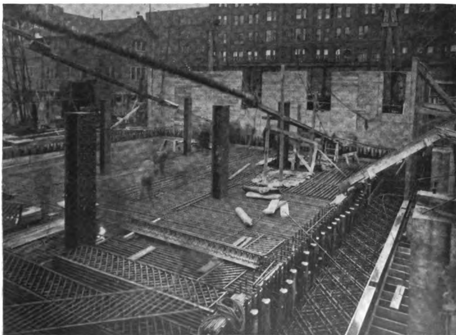
As the steel re-inforcing for the main vaults of the Federal Reserve Bank of Cleveland, Ohio, looked during construction. This installation was by the Rivet-Grip Steel Company, Cleveland, Ohio
