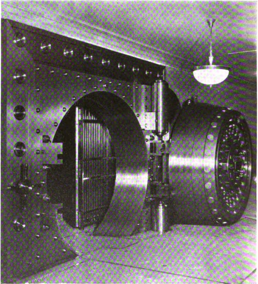
Main entrance to the safe deposit vault of the Illinois Trust Safety Deposit Company, Chicago. Vaults and entrances built and installed by
