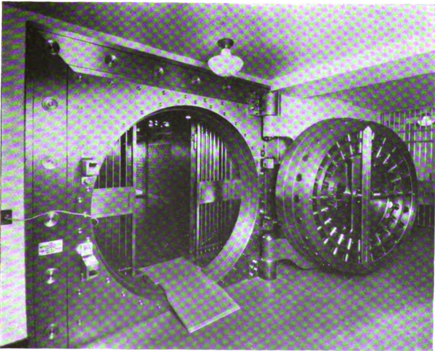
Main entrance to the safe deposit vault of the Bishop Trust Company, Limited, Honolulu, T. H., built by the York Safe & Lock Co., York, Pa. The vault has 2000 safe deposit boxes and a capacity of 6300. The 23-ton door is the largest safe door ever brought into the Hawaiian Islands.
