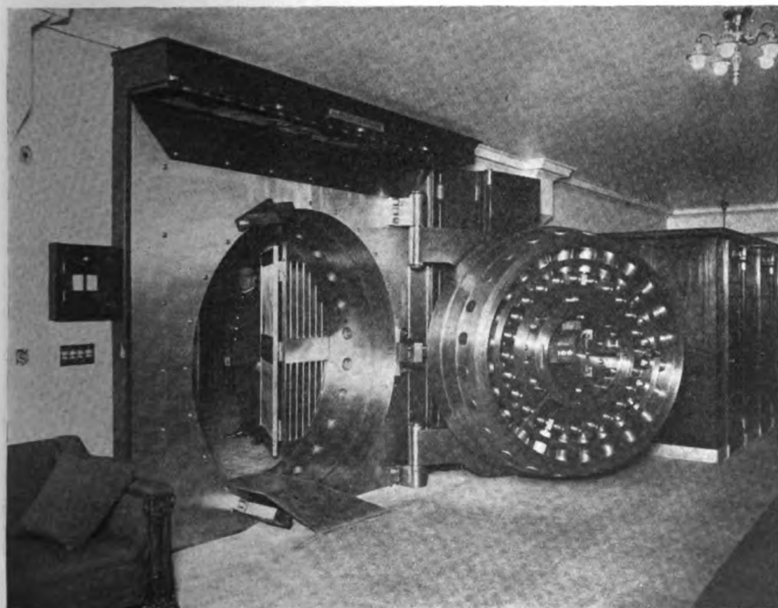
Safe deposit and security vault, Seventy-third street branch, United States Safe Deposit Company, New York. Designed, manufactured and installed by Herring-Hall-Marvin Safe Co., Hamilton, O., and New York, N. Y.
