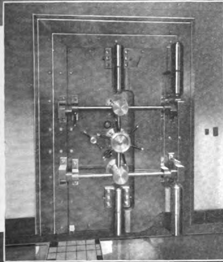
Vaults and Equipment of National City Bank of New York, Havana, Cuba.
