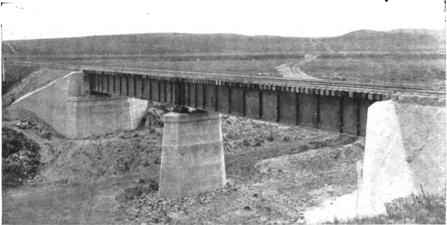
STEEL BRIDGE, CONCRETE FOUNDATIONS, ON THE YELLOWSTONE DIVISION OF THE NORTHERN PACIFIC RAILWAY
