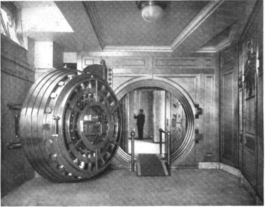
VAULT, UNION TRUST COMPANY, SAN FRANCISCO, CAL. DOOR OPEN SHOWING BOLT WORK AND FOOT BRIDGE
