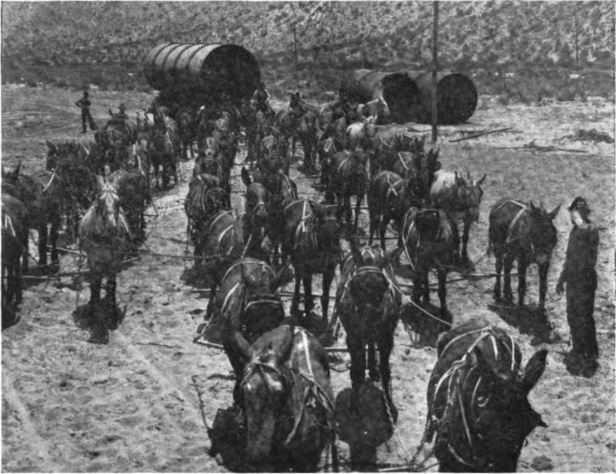
SECTIONS OF THE GREAT SIPHON WERE HAULED FROM THE RAILROAD STATION, SEVEN MILES OVER SANDY ROADS IN SPECIALLY CONSTRUCTED WAGONS DRAWN BY FIFTY HEAD OF MULES.
