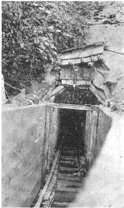
LOOKING THROUGH TUNNEL NO. 11, WHICH IS 1900 FEET LONG, DRIVEN STRAIGHT THROUGH A MOUNTAIN OF SOLID GRANITE. THE WHITE SPOT IN THE CENTRE OF THE ARCH IS THE PORTAL AND REFLECTION AT THE OPPOSITE END
